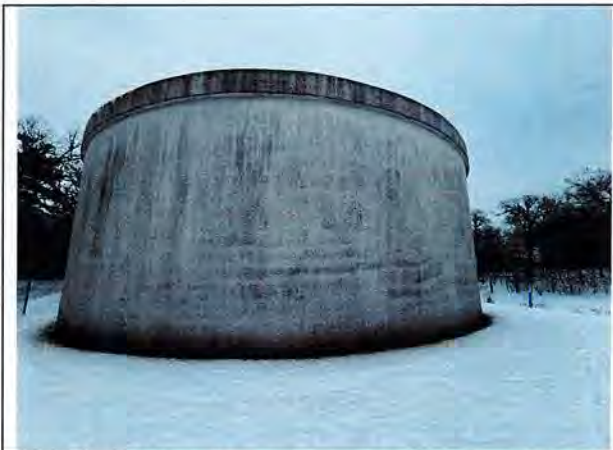
500,000-gallon ground tank owned by MHOG
