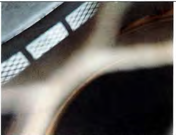
Vent screen has fallen into tank
