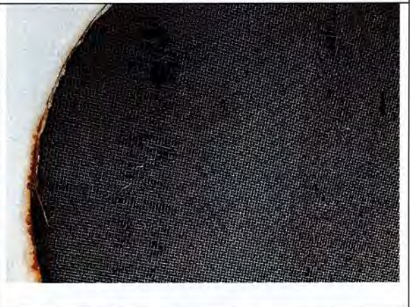
Holes in overflow screen
