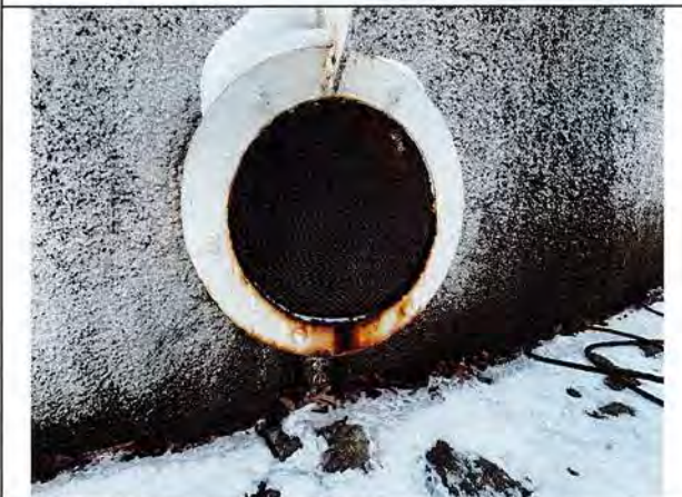
Overflow pipe with 24 mesh screen
