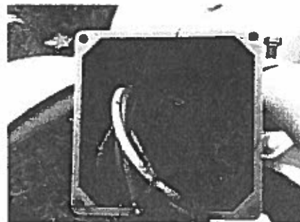
Picture of inside the junction box
